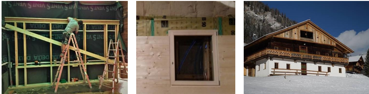
figure 9: left: Black wind paper and the frame construction for the OSB panels in “Hof Neuhäusl” © DI Hans Peter Gruber; right: New block wall on the inside of the “Giatlahaus”. The space between the old log wall and new log wall was insulated with sheep wool. ©Benjamin Schaller
