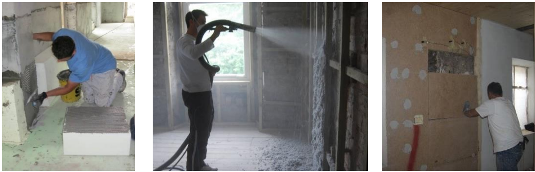
figure 2: left: installation of internal insulation (Perlite) at Villa Castelli © Eurac; middle: Blowing on the wet cellulose insulation material © HES; right: installation of wood fibre © Eurac
