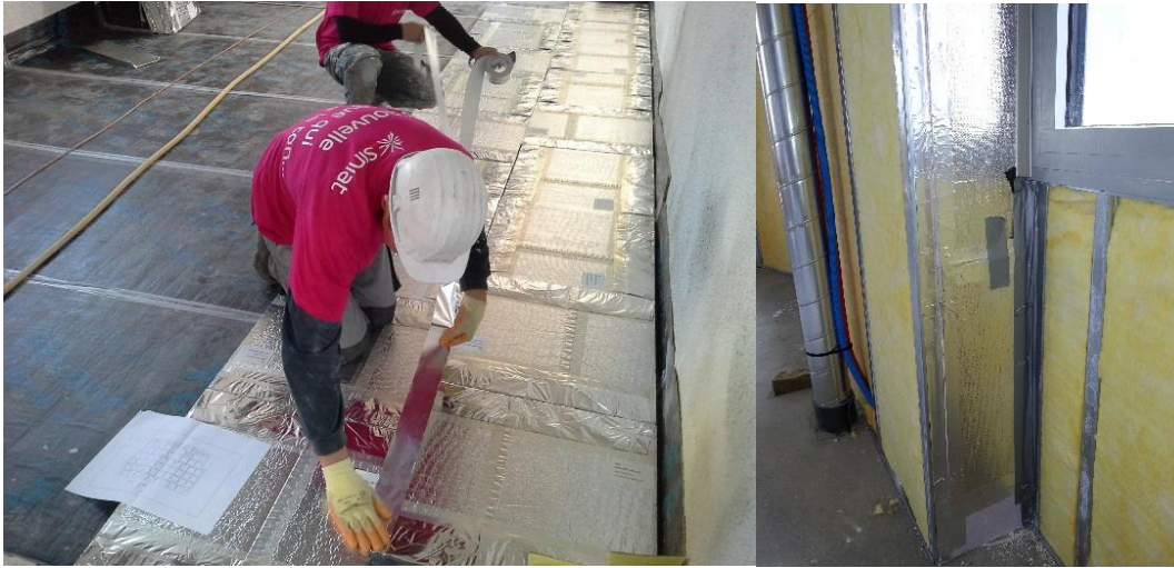
Figure 3-18: Building in Nantes insulated with VIPs in floor and on the interior of the existing walls (Photo: POUGET Consultants).
