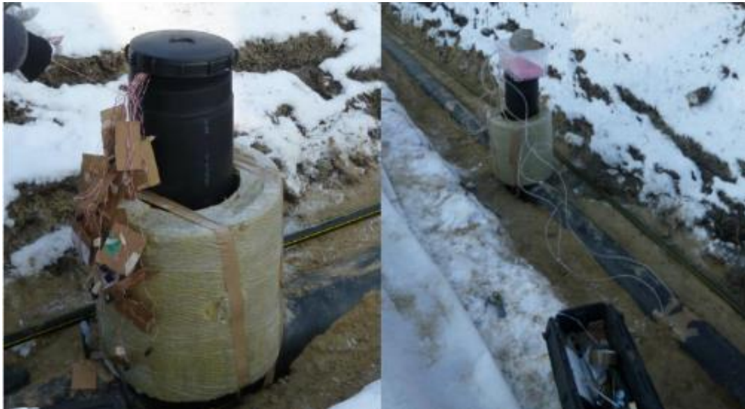
Figure 3-17: District heating pipes monitored in field (Photo: Axel Berge).
