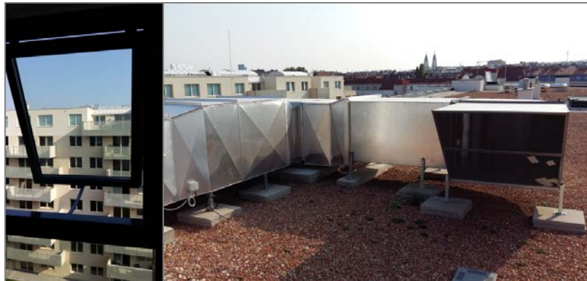
Figure 49 Ventilative cooling components: air inlet window, air exhaust unit with ventilator on roof.
