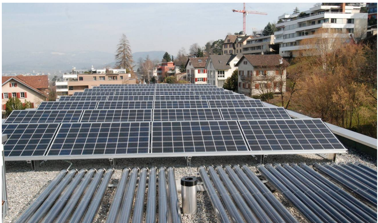
Figure 11: Thermal and PV-collectors on the roof reduce the yearly energy consumption close to zero
