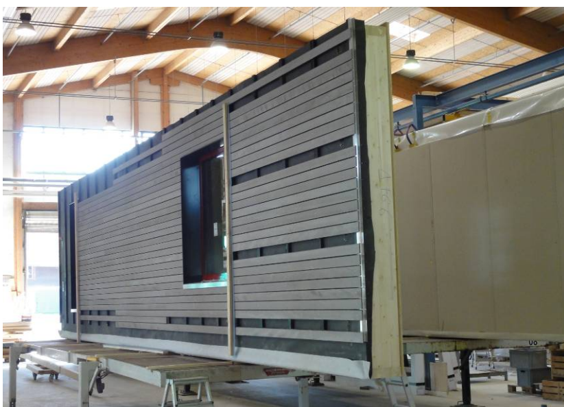
Figure 15: The windows and the wood cladding are installed, except for areas where the module has to be fixed on site
