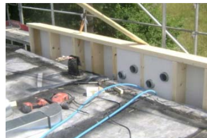
Figure 21: The step back of the penthouse floor is used for the horizontal ventilation distribution
