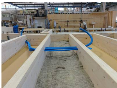
Figure 10: Ventilation pipes and electric conduits are integrated into the modules.
