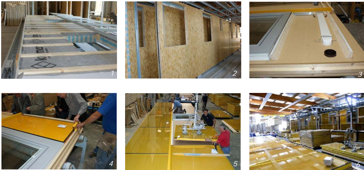
Figure 16: Sequence of prefabrication procedure in the fabrication hall (Source pictures 5-6: Gap-Solution GmbH)
