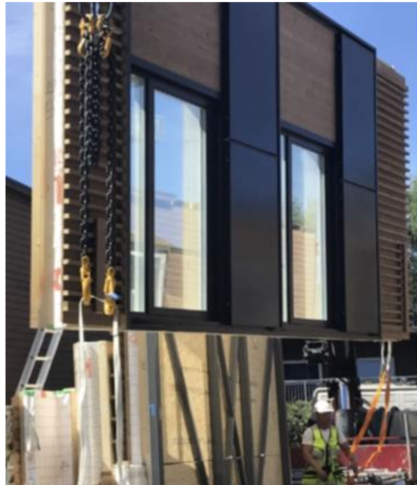
Figure 59. Prefabricated facade elements with BIPV panels being installed during a deep retrofit project in Hagerud-senteret. Photo taken during the EU-prosjekt 4RinEU (Grant agreement ID: 723829). Prefab modules and design by Lindal Hus and Filter Architects. The building is owned by Oslobygg (formerly Boligbygg). [5].
