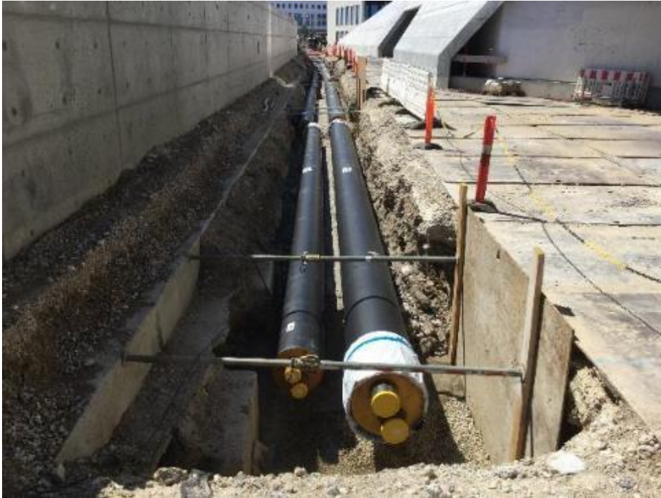
Figure 34. District heating pipes to a large customer (Source: Taarnby Forsyning and Ramboll).
