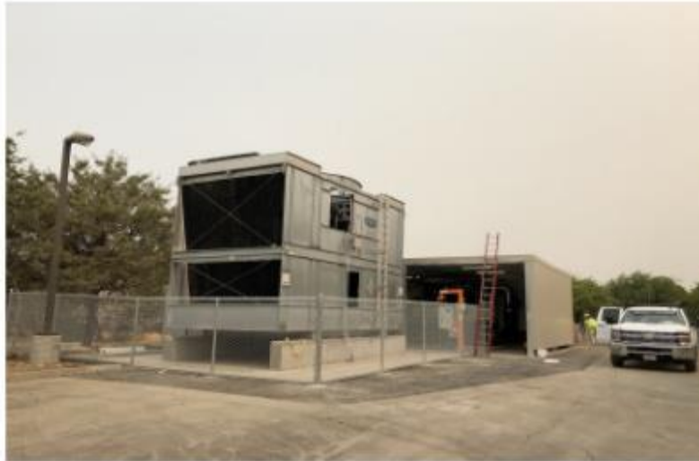
Existing Chiller at Primate Center
