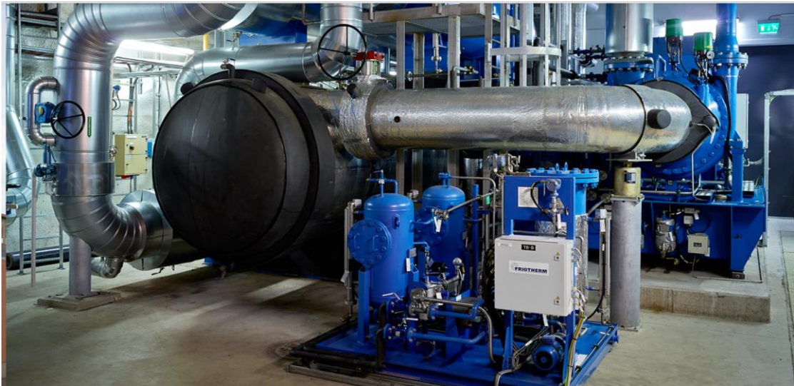
Figure 107. Katri Vala facility (Source: Helen).
