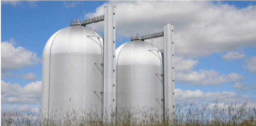
Figure 52. Heat storage tanks at Avedøre CHP plant (Source: Ramboll).
