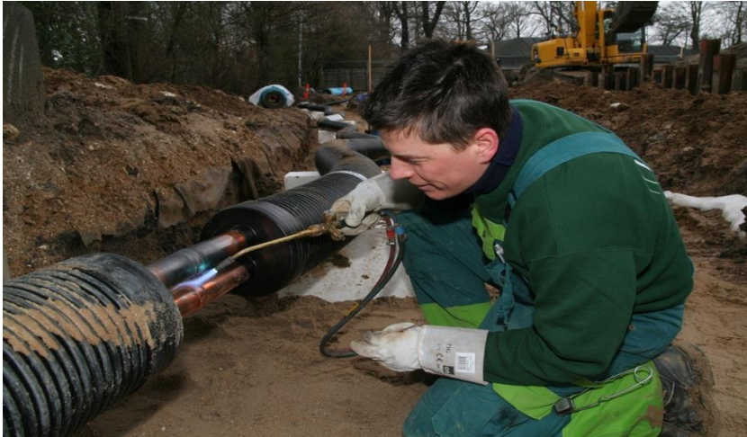
Figure 46. Installation of preinsulated twin pipes of supply of small buildings (Source: Ramboll).
