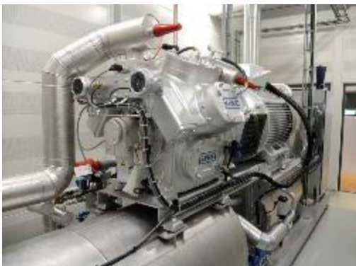
Figure 76. One of the installed 500 kW heat pumps (Source: Danfoss).
