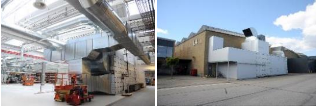
Figure 75. Left: large ventilation system installed in the production halls to collect exhaust heat from machinery; right: main ventilation system (Source: Danfoss).
