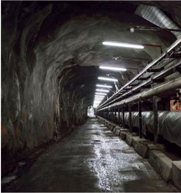
Figure 110. Underground facility (Source: https://www.helen.fi/en/news/2018/Construction-of-rock-cavern-heat-storage-facility-starts/ ).
