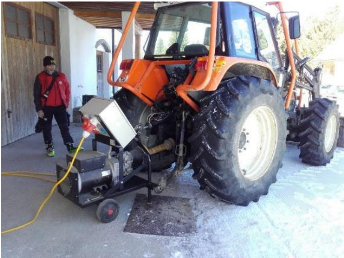
Figure 7. Tractor providing power to a mountain resort during 3-hour blackout. This is a typical mobile backup method used in agricultural and sparsely populated areas (February 2020, Sommeralm in Austria. Source: AEE INTEC).
