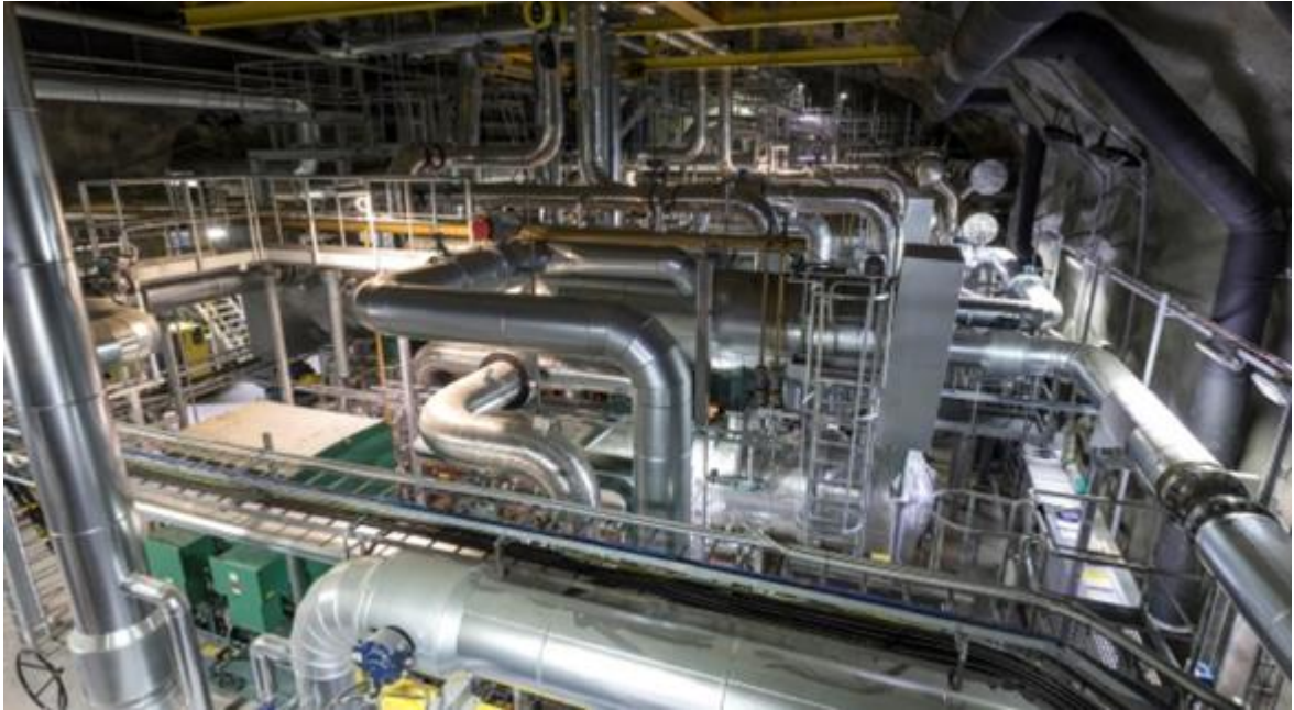
Figure 105. New heating and cooling plant located under Esplanade Park at a depth of 50metres (Source: Helen).
