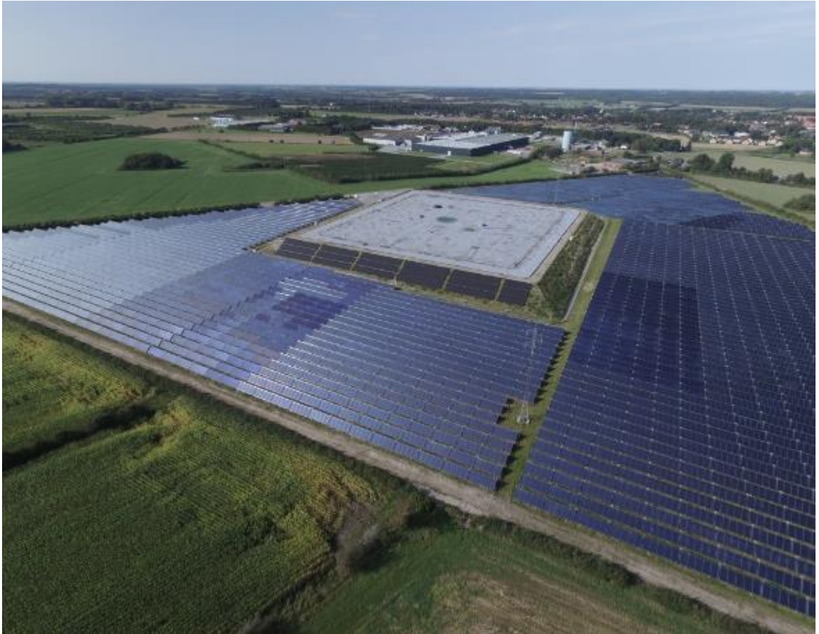
Figure 84. Gram district heating solar heating and heat storage pit (Source: Gram Fjernvarme).
