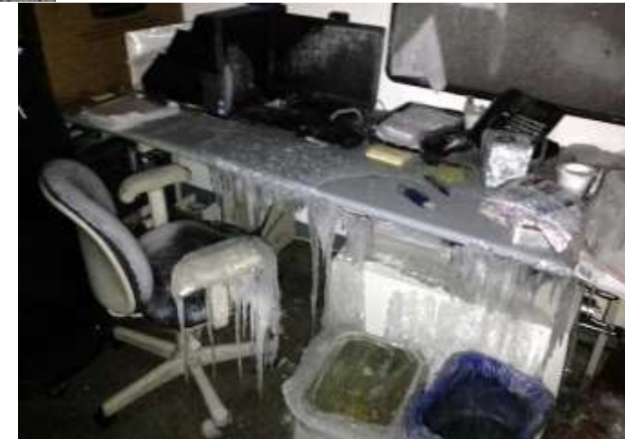
Frozen water pipes, damaged furniture and other property, jeopardized mission
