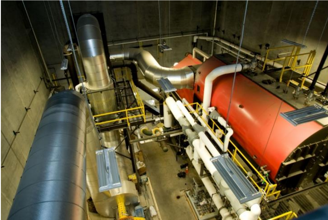
800 horsepower biomass boiler making steam at 400psi
