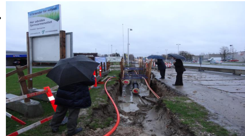
4TH GENERATION DISTRICT ENERGY 06-12-2017
